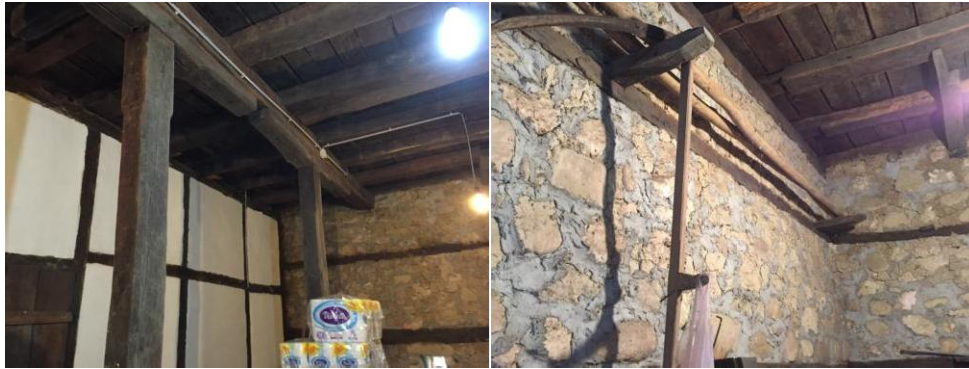
Figure 17: Structural assembly of the house visible from the ground floor Source: Author (07.22.2016.)
